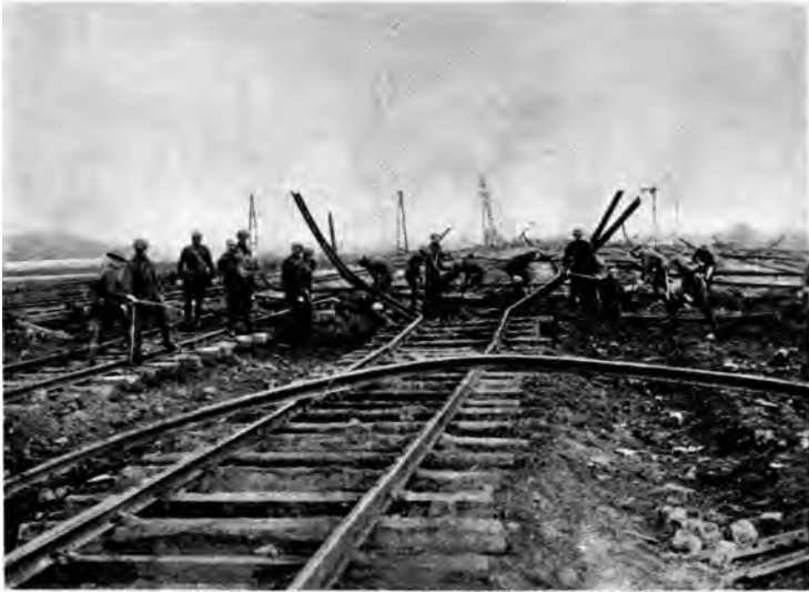
View of destroyed railroad tracks at Waereghem, Belgium. These tracks were destroyed by mines before the Germans retreated from the city. Men working in picture are from Company A, 316th Engineers.
